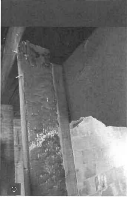
Fire Damage to beams and 1 st floor Flooring
